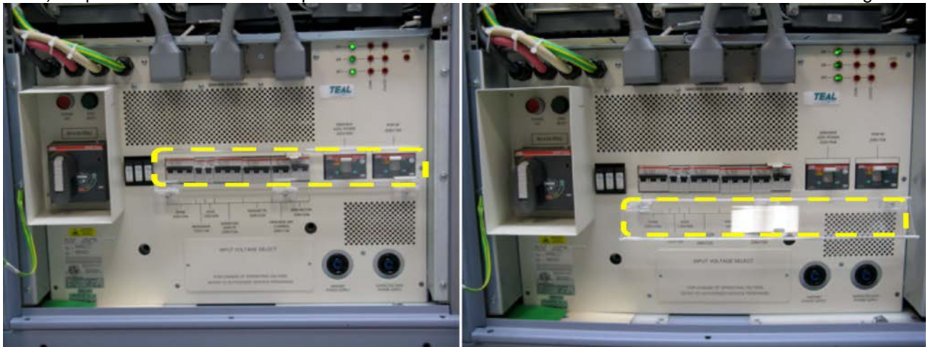
Figure 1. Clear plastic cover closed (left) and open (right) that protects circuit breakers in PDU.
