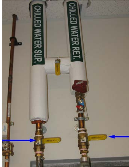
Figure 5. Chilled Water Supply and Chilled Water Return. Verify valve position (closed) in the Equipment Room
