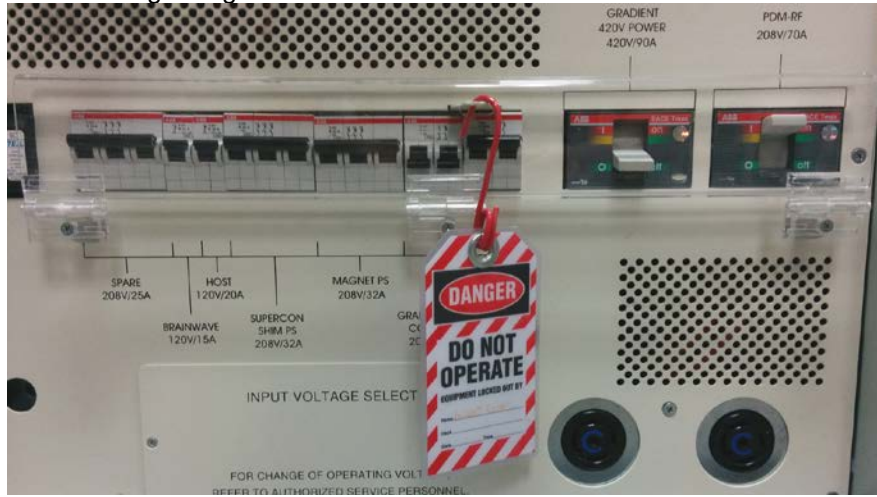
Figure 3. Use lockout tag when gradient amplifiers are off and while switching gradient cables
