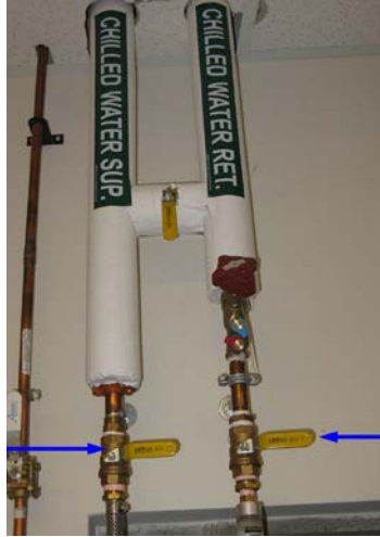
Figure 27. Chilled Water Sup. and Chilled Water Ret. Verify valve position (closed) in the Equipment Room.
