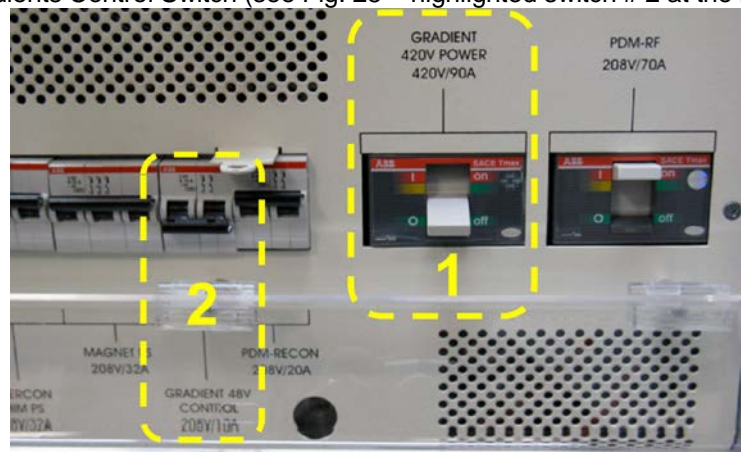
Figure 25. Turn the circuit breakers off in the following order: 1 st - “GRADIENT 420V POWER 420V/90A” 2 nd - “GRADIENT 48V CONTROL 208V/10A”
