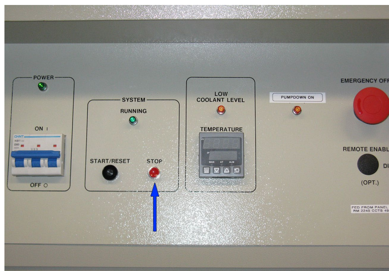
Figure 21. Turn off chiller if Spinmaster not in use.
