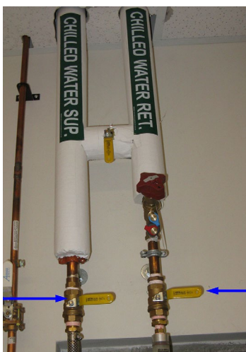
Figure 22. Chilled Water Sup. and Chilled Water Ret. Verify valve position (closed) in the Equipment Room.
