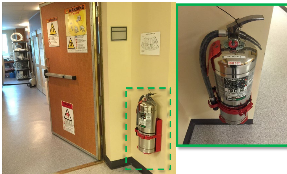
Figure 2.1 non-magnetic fire extinguisher
